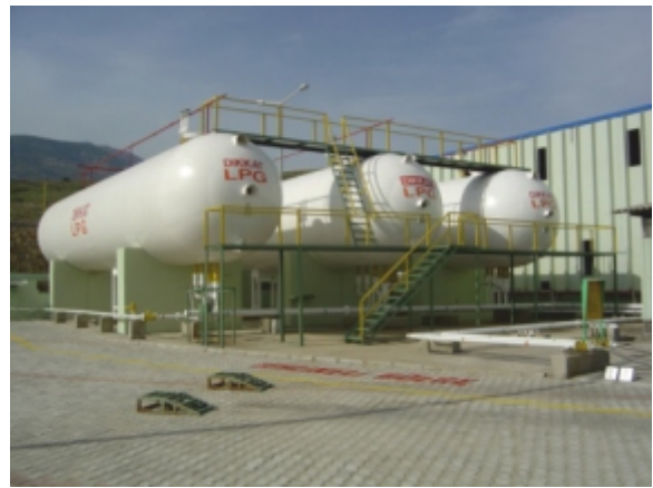
LPG Storage Tanks Application
