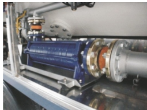
Model No: PSC 5006 Skid System Application Road Tanker Unloading Pump
